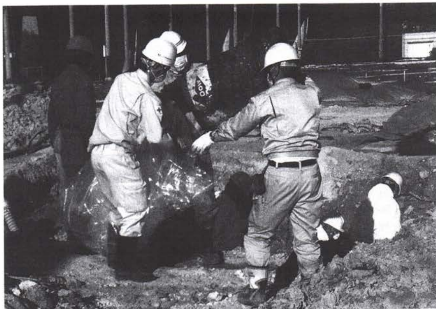
A construction crew unearths a chemical barrel on an Okinawa City soccer pitch in January 2014. Photo by Kuwae Naoya
